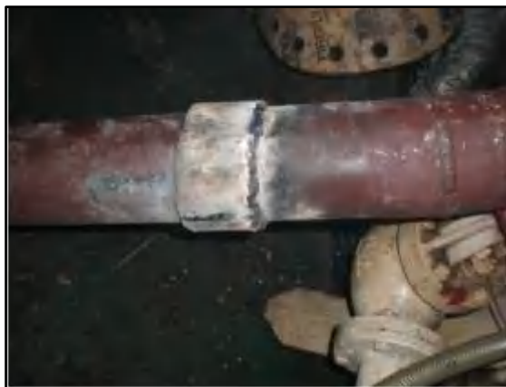
Gambar 8. Galvanic corrosion ( Budi Utomo,2009 )
