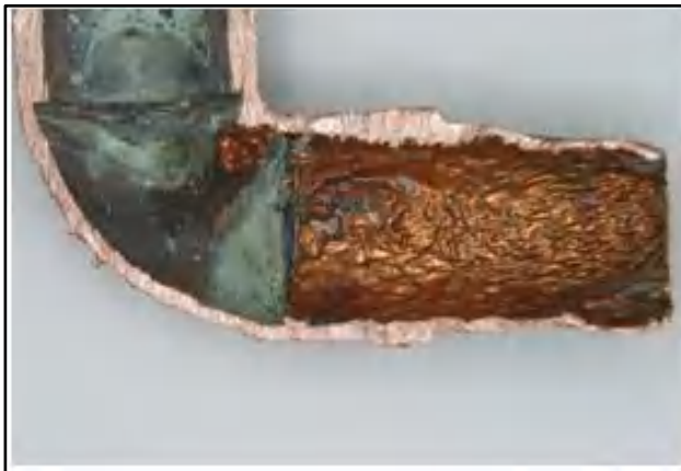
Gambar 7. Errosion corrosion ( Budi Utomo,2009 )
