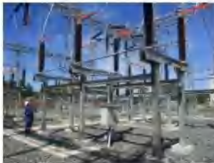
Gambar 3. Disconnecting Switch Sumber: Affif A., 2018
