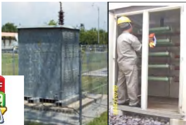
Gambar 18. Neutral Grounding Resistor (NGR) (Sumber: PLN, 2024)
