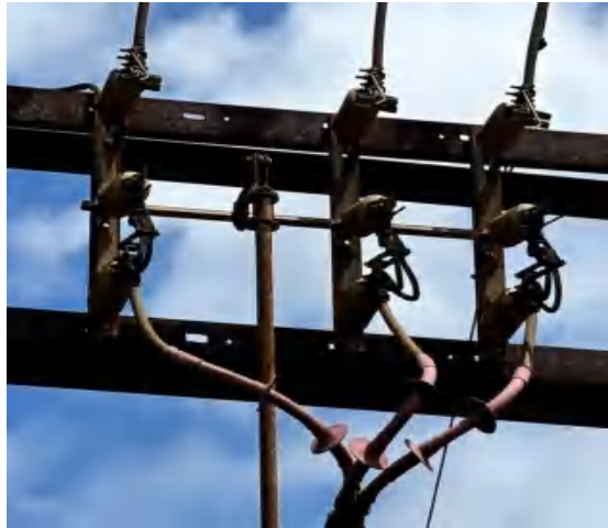
Gambar 12 Disconnecting Switch (DS)
