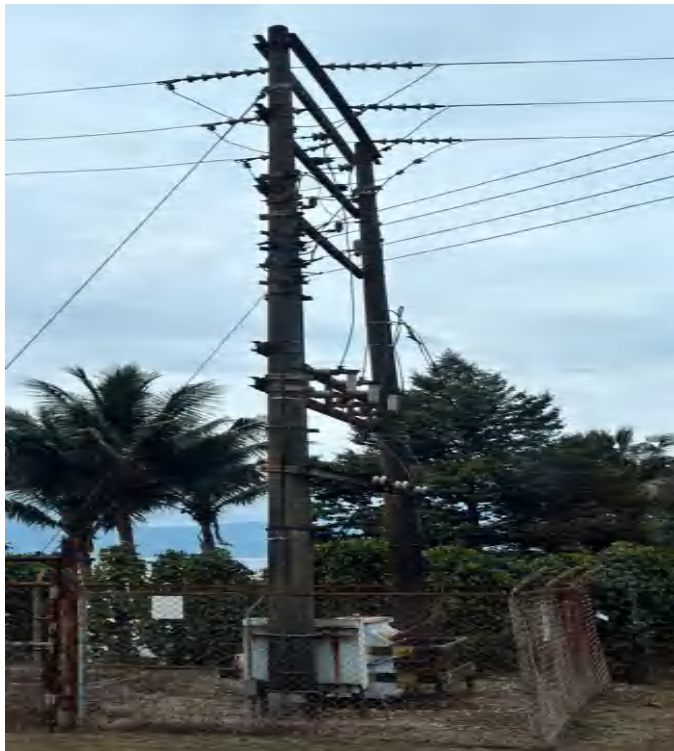
Gambar 7 Gardu Distribusi Sumber: PT. Vale Indonesia Tbk
