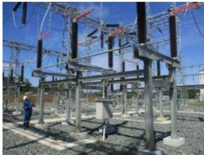
Gambar 3. Disconnecting Switch Sumber: Affif A., 2018
