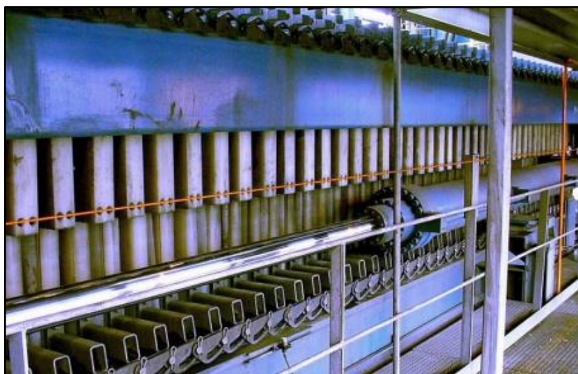
Gambar 11. VPA (vertical pressure air blow)
