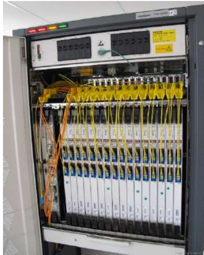
Gambar 3 Optical Line Terminal
