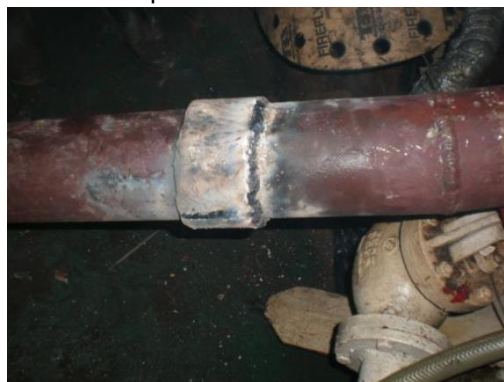
Gambar 4 Galvanic corrosion (Sumber: B. Utomo, 2012)
