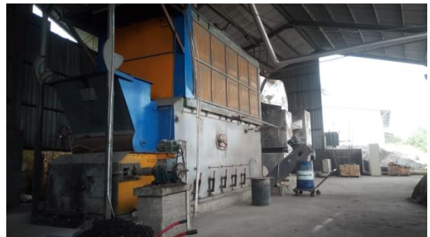
Lampiran Gambar 6. Mesin Boiler
