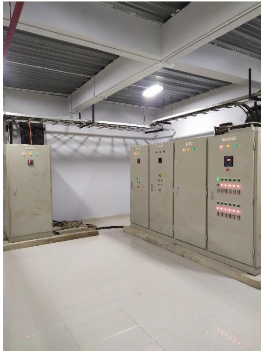
Lampiran 1 Ruang Panel Incoming PLN
