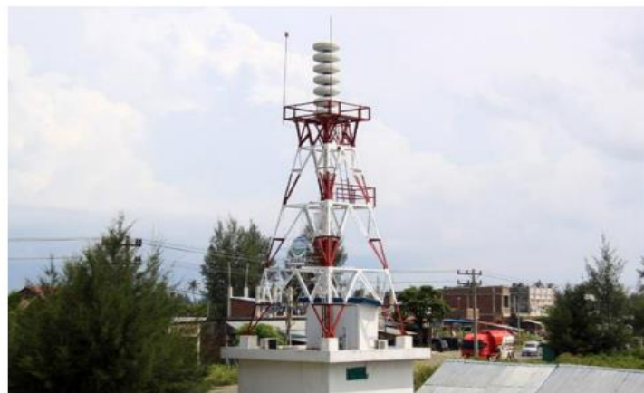
Gambar 11 Menara sirene Tsunami
