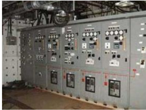
Gambar 2.1 Main switch board pada kapal (Sumber: www.marineengineeringonline.com )
