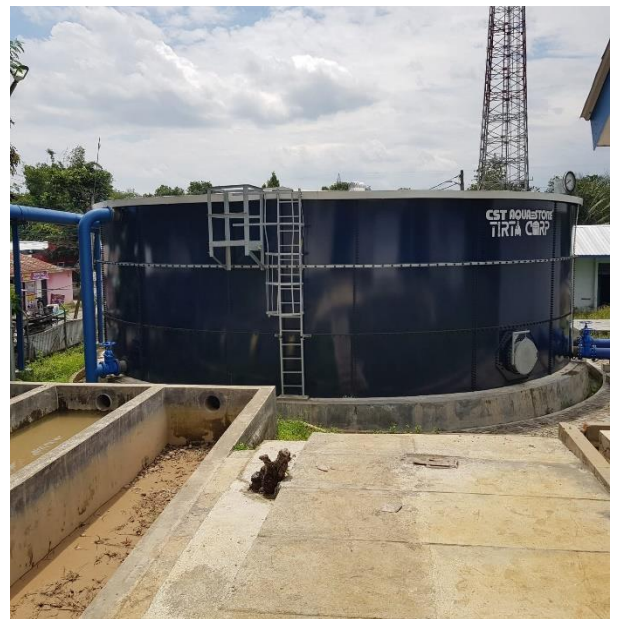
Bak Unit Penampung (Reservoir)
