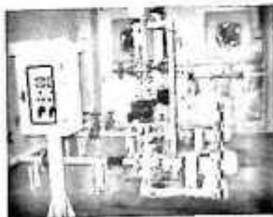
Pompa Gas Klor
