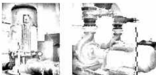
Pompa Air baku Intake II Mallengkeri
