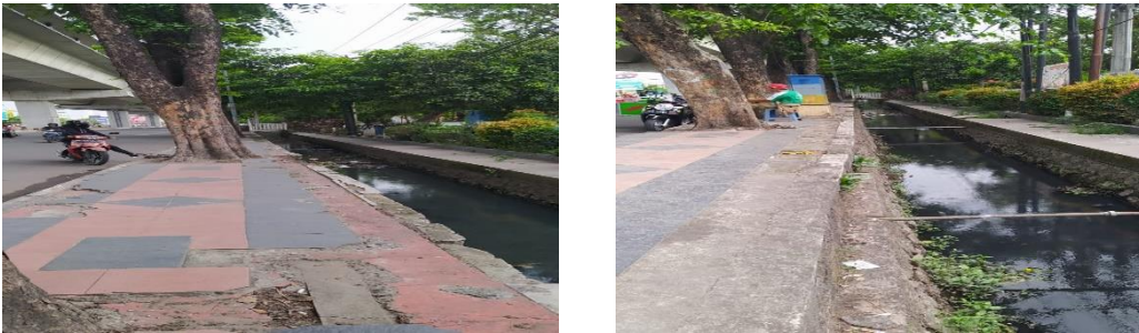
Figure 1. The condition of the pedestrian path on Jalan Andi Pangeran Pettarani
