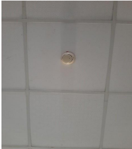
Gambar 2.4. Smoke Detector Sumber: Data Primer, 2020
