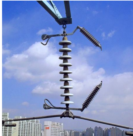
Gambar 15 Transmission Line Arrester (Giraudet, 2022)
