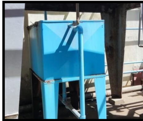
Gambar 2.9 Feed Water Tank
