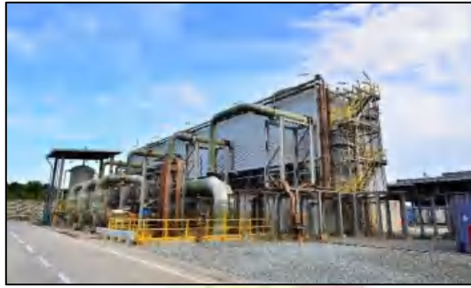
Lampiran Gambar 17 Instrumen Sea Water Cooling Tower
