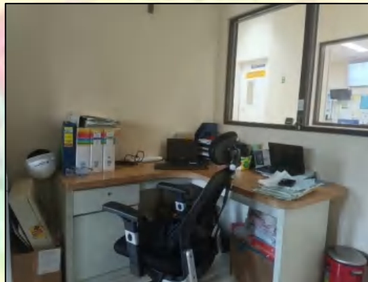
Lampiran Gambar 24 Ruang Data DCS (Distribution Control System)
