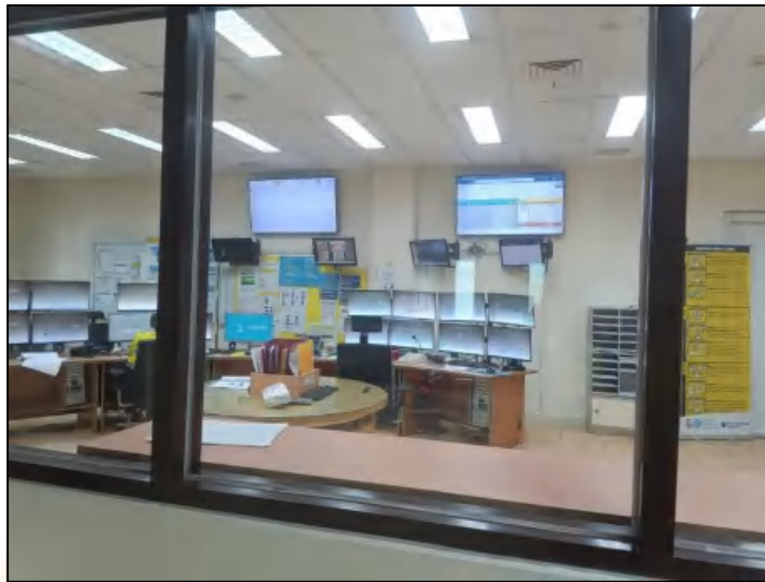
Lampiran Gambar 23 Ruang DCS (Distribution Control System) 1
