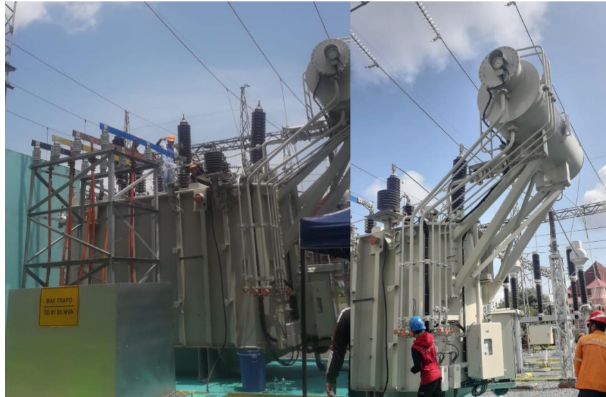
Gambar 4 Transformator daya 60 MVA GI Panakkukang
