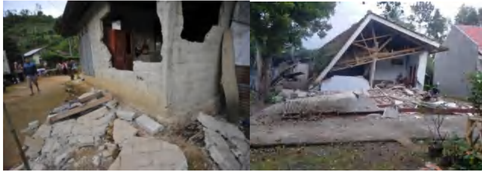
Gambar 2.2 Kerusakan non-engineering building akibat gempa
