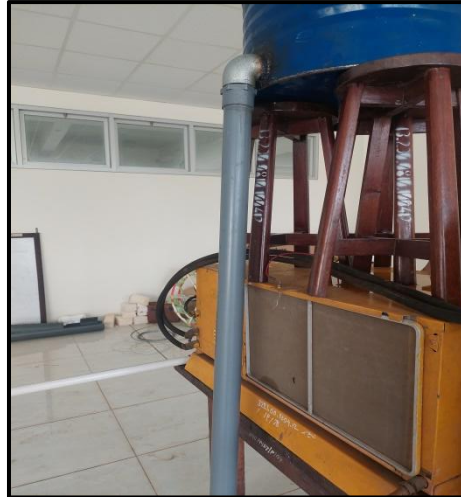
Gambar 28 Pipa pvc 2 inch
