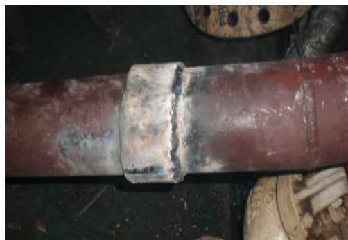
Gambar 4. Korosi galvanis ( galvanis corrosion ) (Utomo, 2009)
