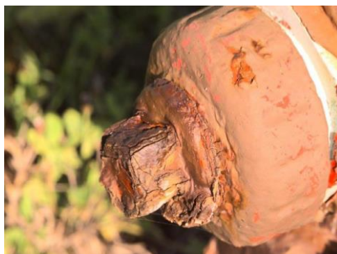
Gambar 8. Korosi lelah ( fatigue corrosion ) (Utomo, 2009)
