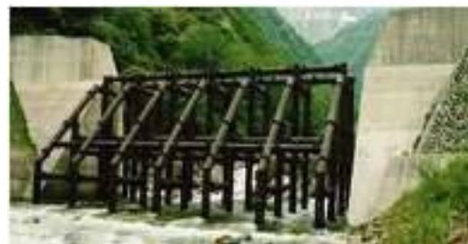
Gambar 5. Check Dam Tipe Grid
