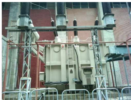
Gambar 2.9 Transformator PLTA Bakaru I (Bakaru HPP, 1990)
