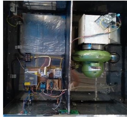
(b). Hardware sistem kontrol
