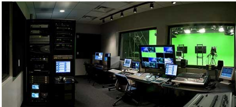
Gambar 2.12 Ruang Production Control Room
