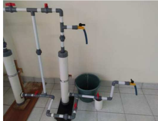
Gambar 19. Proses back wash (pencucian balik)
