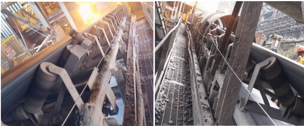
Belt Conveyor 2BC 3B di North South Mill, PT. Freeport Indonesia
